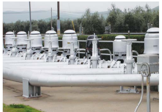
Figure 2. Irrigation pumps deliver water to customers in the higher elevations to the east of the canal.
