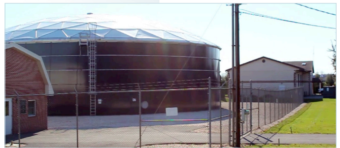
Middlesex Township needed to improve communication from several remote sites, such as this water tank.
