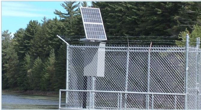
In locations with no line power, solar panels power the radios.
